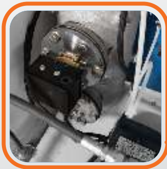
Controllo livello acqua in caldaia mediante galleggiante. Water level control in the boiler by means of a float.
